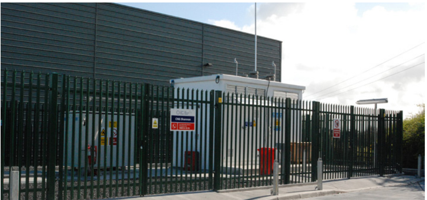
Figure 6-3: Clean Ireland Recycling CNG Facility
