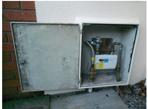
The meter box and area surrounding the meter prior to service renewal.
