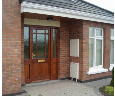
Example of a meter box in an area with the potential to be enclosed.
